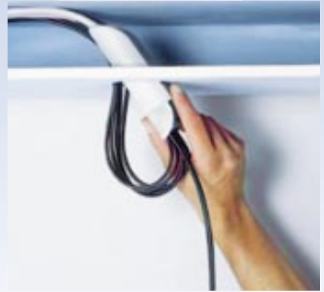
The HALOTRONIC MOUSE® is easily inserted through a ceiling cut-out for a downlight
