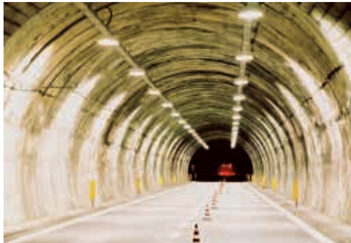
Fig. 2. Thirty five 150 W ENDURA lamps illuminate the tunnel between Genua and Ventimiglia
